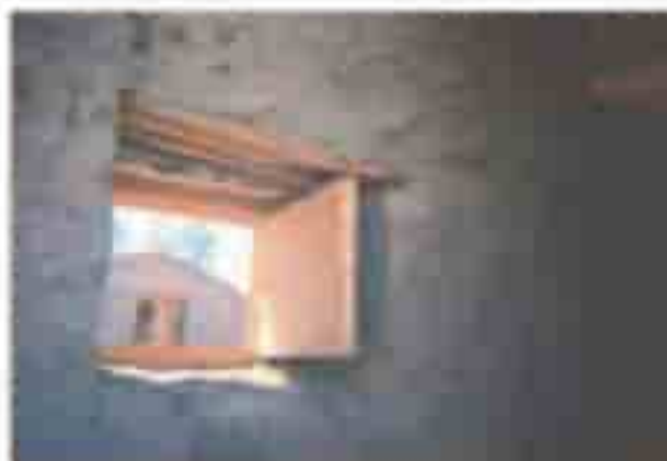
Picture No. 7: Installed wall ventilator
